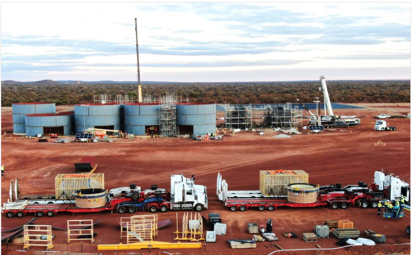
Figure 1: Delivery of the mill motors (63 tonne, 9000kW each) and trunnions (44 tonne each) to KOTH, with the construction of the CIL tanks and the Mill plinths in the background.
